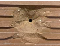
Hammer action drilling resulting in blowout and microcracking.
