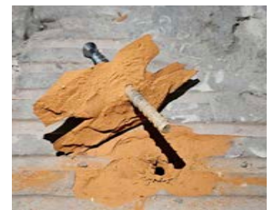
Typical tension failure mode in HCT.
